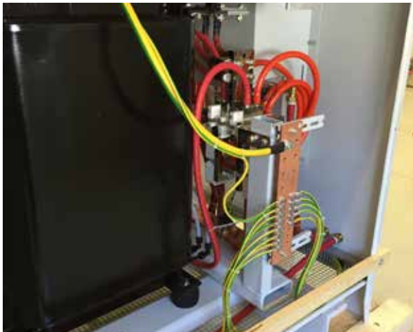
Thyristor controlled transformer
